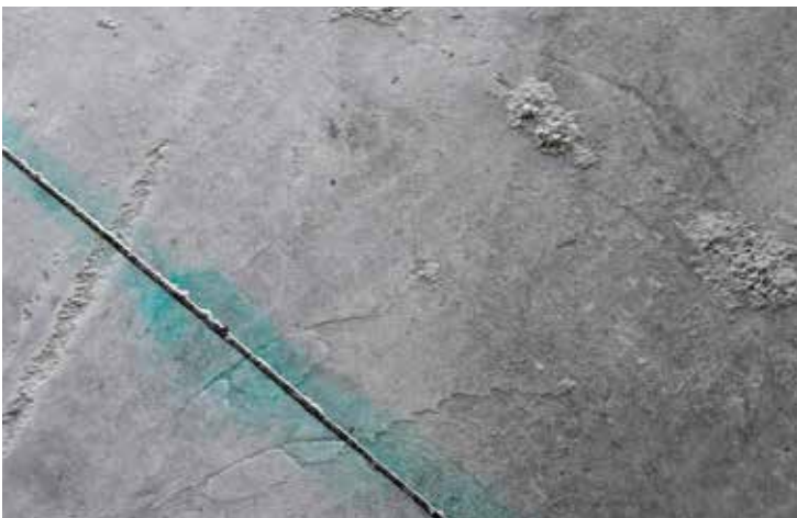
Surface defects due to bad finishing.
