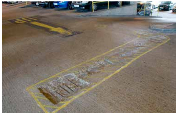
Aggressive chemicals degrade concrete. The picture shows damages of chloride attack from de-icing salts.
