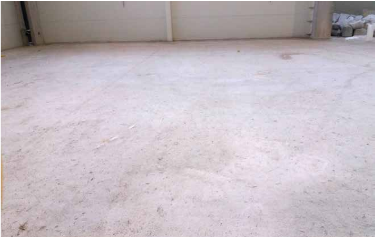
Delaminated dry shake hardener floor after substrate preparation.
