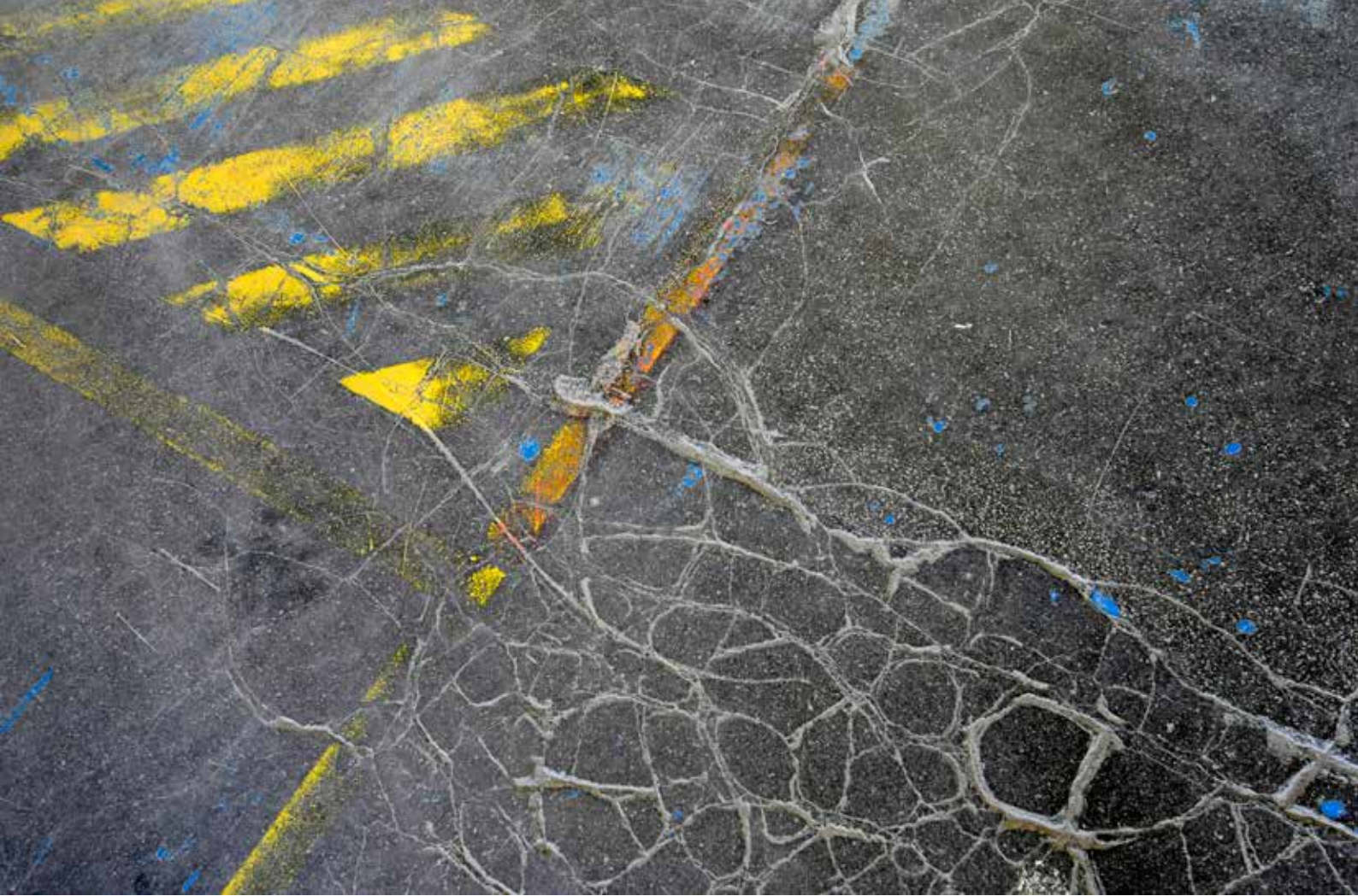
All cracks are not the same. Before repair remedies the cause of the cracks should be clarified.
