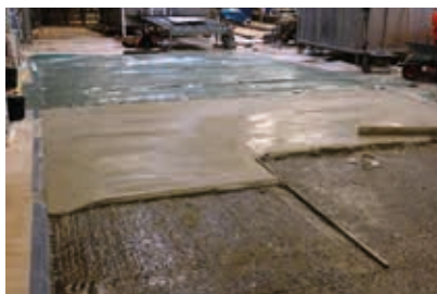
FRIDAY EVENING: Application of the bonding layer and the cementitious fast curing Sika® Ucrete® UL flooring screed.
