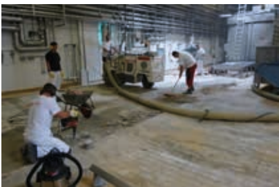
FRIDAY AFTERNOON: Mechanical removal of old tiles and epoxy adhesive. Substrate preparation and cleaning.
